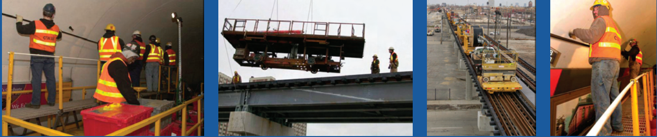
Left: Electricians work on fiber optics installation. Center: The Aldridge team used a cable car to transport supplies. Right: The logistics of working near electrified rail is a challenge.
